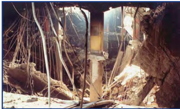
The resilience of a column in the aftermath of the 1993 World Trade Center attack.
